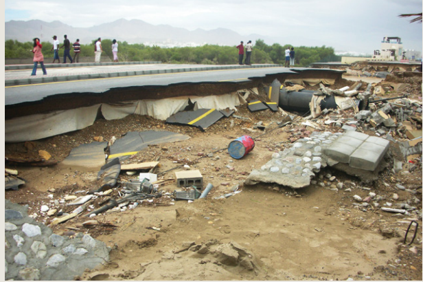
Damages in Muscat after the passage of Cyclone Gonu, Oman, 2007. Source: Wikimedia Commons.
